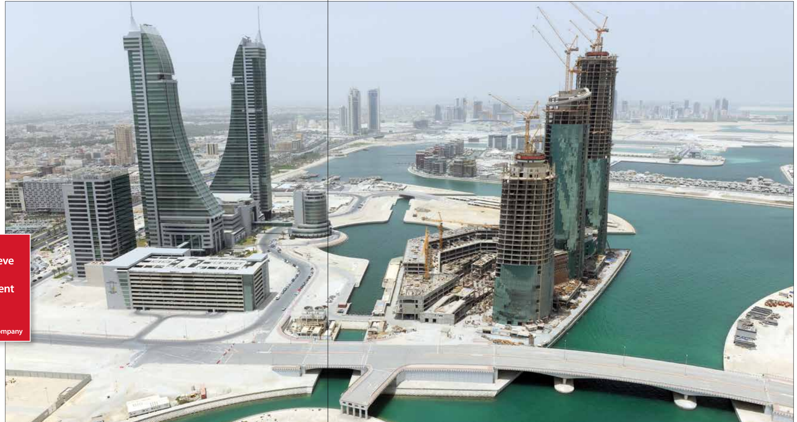
Ready to go: the Villamar structure and site equipment has been certified as sound ready for work to restart
